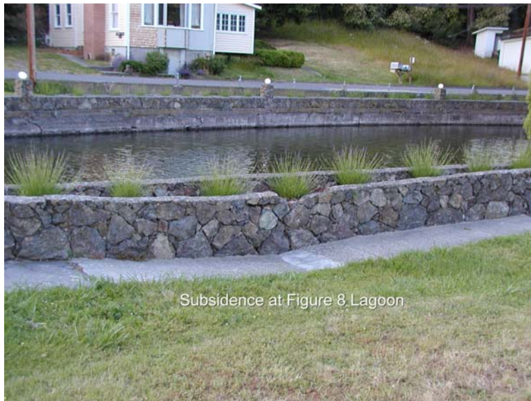
The existing wall and sidewalk have settled probably because of decay of organic material or compaction of very loose sediments.
