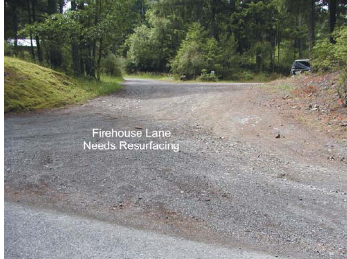
Existing roads cut directly into native earth, without the placement of a gravel mat or asphalt pavement, are a source of turbid stormwater runoff.
