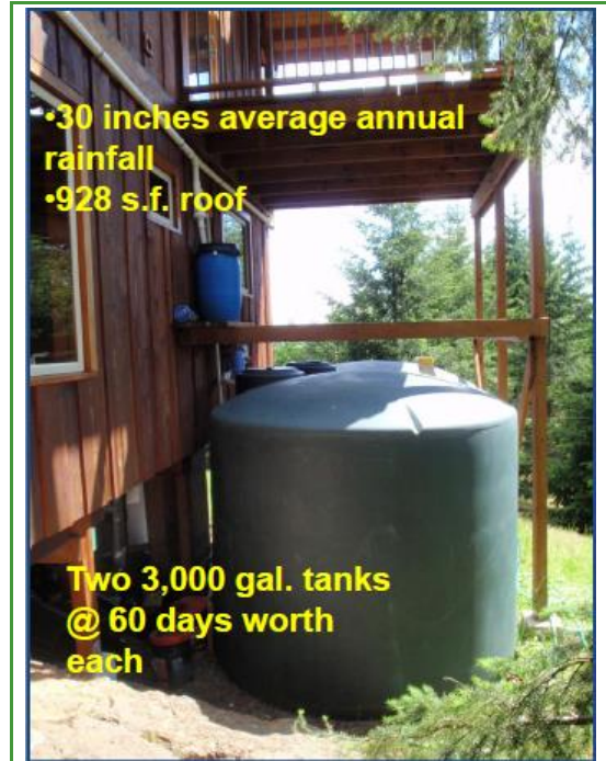
Figure 14. Residential Cisterns for Storing Rainwater Stored Under a Deck.
