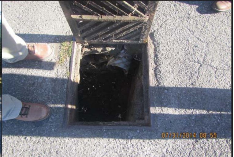
Partially clogged catch basin on School Road
