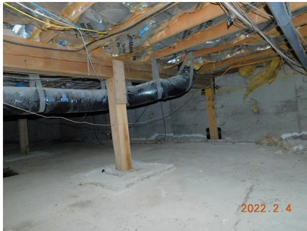
Figure 29. Posts supporting the first floor framing bear on concrete footings with no mechanical connection to the footing. Plywood gussets can be seen connecting the beams to the wood post (arrow).
