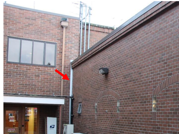
Figure 33. Vertical expansion joint between the exterior wall of the Sheriff's Wing and the exterior wall of the 1980s Courthouse Addition.
