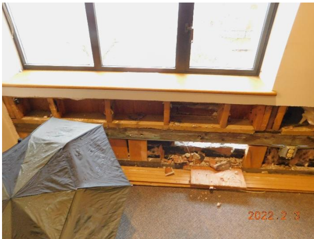
Figure 24. Interior view of the investigation opening on the south wall of the Courthouse Expansion at the interface between the 1980 first level and 1984 second level.
