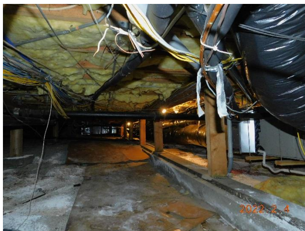
Figure 31. Interior wood-framed cripple wall in the crawl space without sheathing and without anchors into the concrete.
