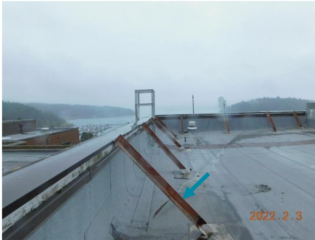
Figure 17. Steel angles (arrows) have been installed to brace the masonry parapet at all four sides.
