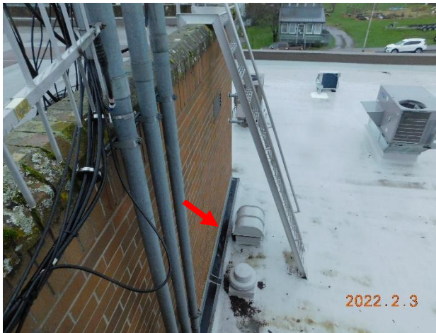
Figure 32. Horizontal expansion joint between the roof of the Sheriff's Wing and the exterior wall of the 1980s Courthouse Addition.
