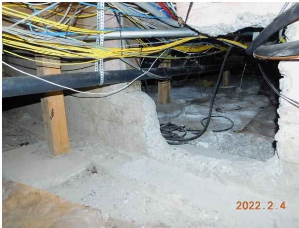
Figure 28. Existing opening previously chipped in the concrete stem wall in the crawl space reveals no reinforcing bars present.
