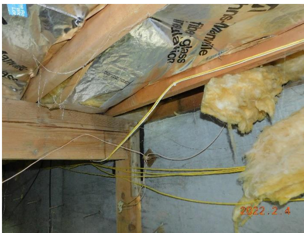
Figure 30. Beam supporting first floor framing for the west side of the building not attached to the interior concrete stem wall.
