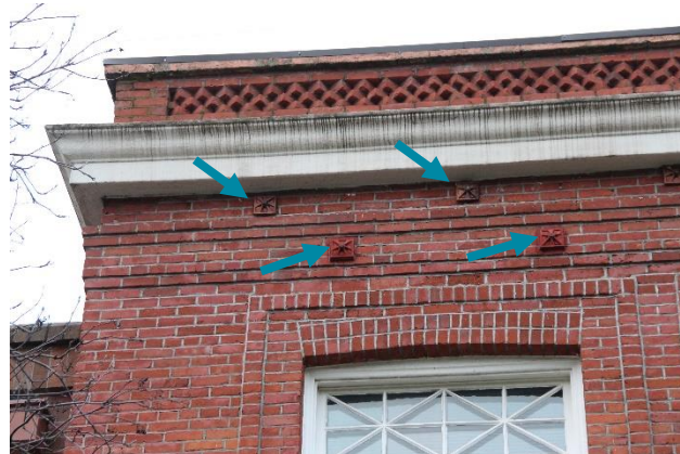
Figure 18. Steel rosette plates (arrows) at the west side of the Courthouse at the roof level.
