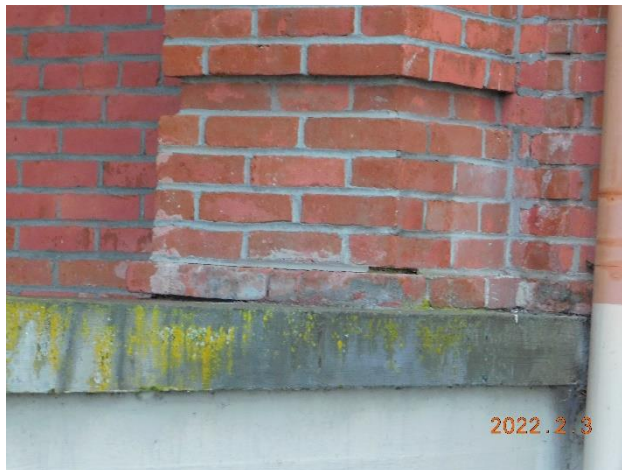
Figure 16. Poorly matched repointing of mortar joints.
