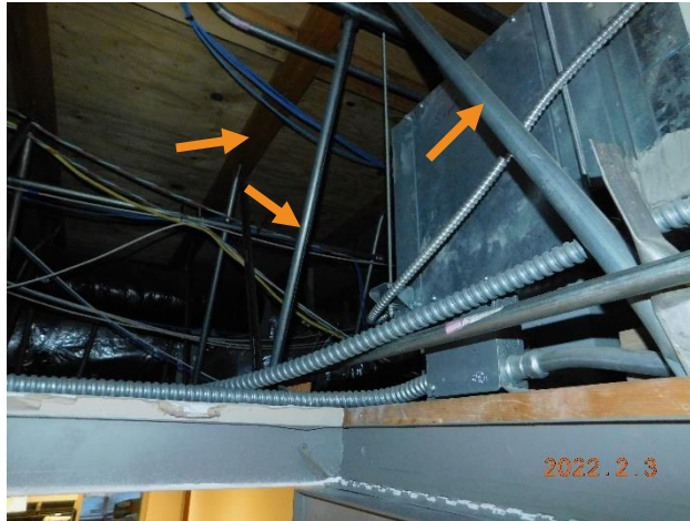
Figure 27. Sheriff's Wing, prefabricated roof truss (Arrows indicate top chord and diagonal members).
