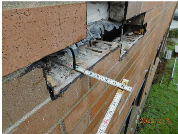
Figure 25. Exterior view of the investigation opening on the south wall of the Courthouse Expansion at the interface between the 1980 first level and 1984 second level.
