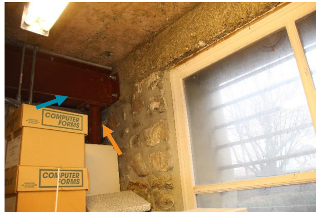
Figure 20. Steel beams (blue arrow) supporting the Level 1 slab are connected to the concrete beam above the stone masonry foundation walls in the basement. The steel beams are also supported by steel pipes (orange arrow) at the perimeter of the basement.
