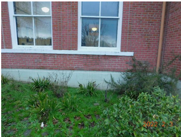
Figure 15. Minor deterioration of exterior brick below the windows.
