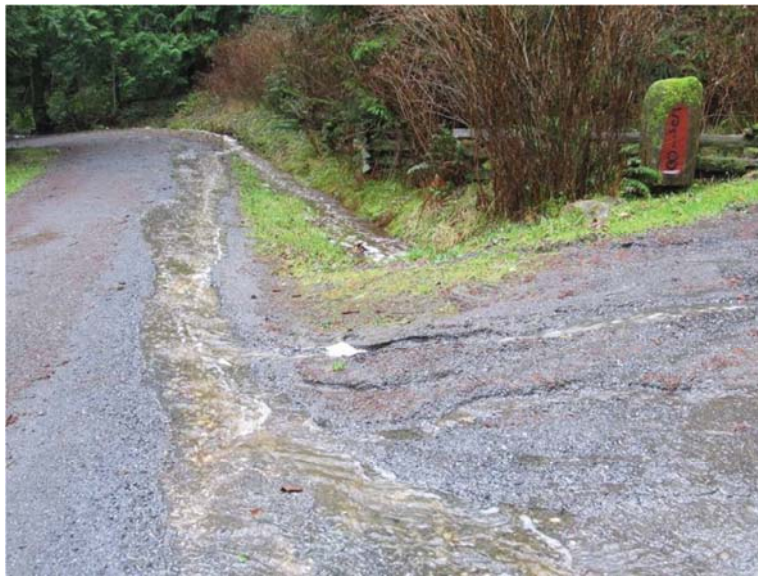
Figure 4. Example of eroding dirt road contributing sediment to the County drainage system (Sutton Road, San Juan Island).
